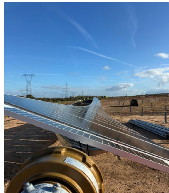
Figure 11: Cibeles Solar Photovoltaic Park | Portugal
