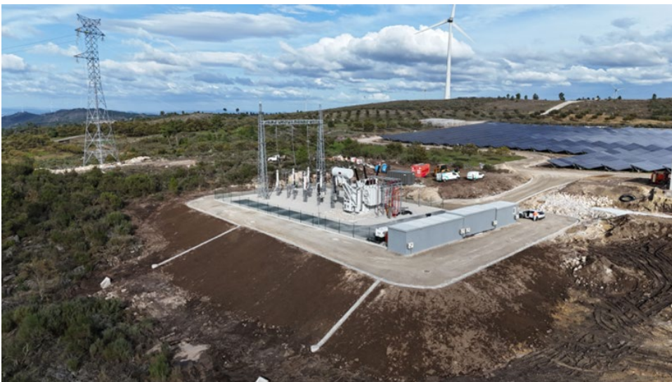
Figure 4: Douro Solar Photovoltaic Park | Portugal
