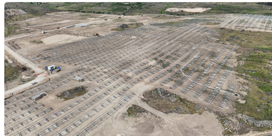
Figure 6: Riodades Solar Photovoltaic Park | Portugal
