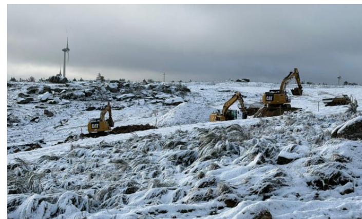
Figure 14: Sendim Solar Photovoltaic Park | Portugal
